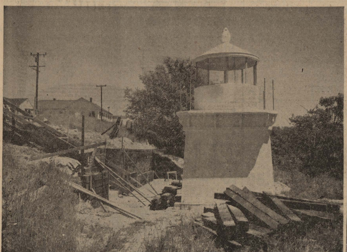
The Trinidad Civic Club has done a nice job with their lighthouse replica. Construction is now under way on a stair from road above.
